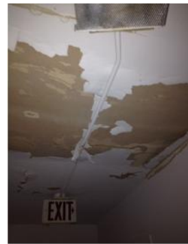
View of peeling white paint.
