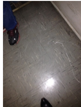
View of 9'x9' asbestos tile.
