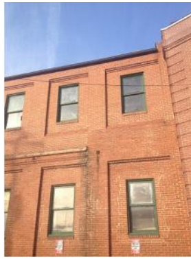
View exterior windows on bldg. 2 same as building 1. Interior color is brown.
