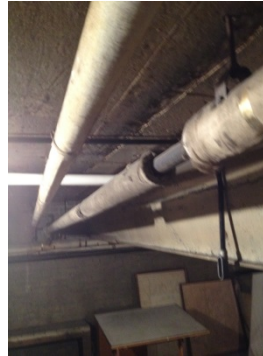
View of asbestos pipe in building 2.
