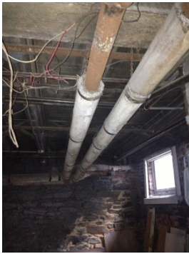
View of asbestos pipe in building 1
