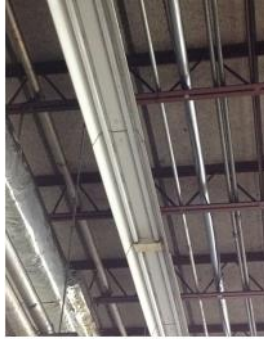
Building 3 Florescent Light Ballast
