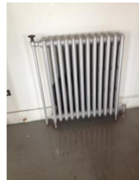
View of radiators
